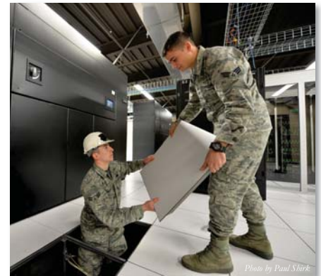
A technician replaces the raised flooring tiles in front of a computer room air conditioning unit.
